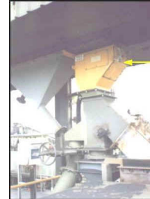
Series 3A style impact weigher with built-in sampler shown with yellow arrow. Sample discharges via small pipe on other side.
